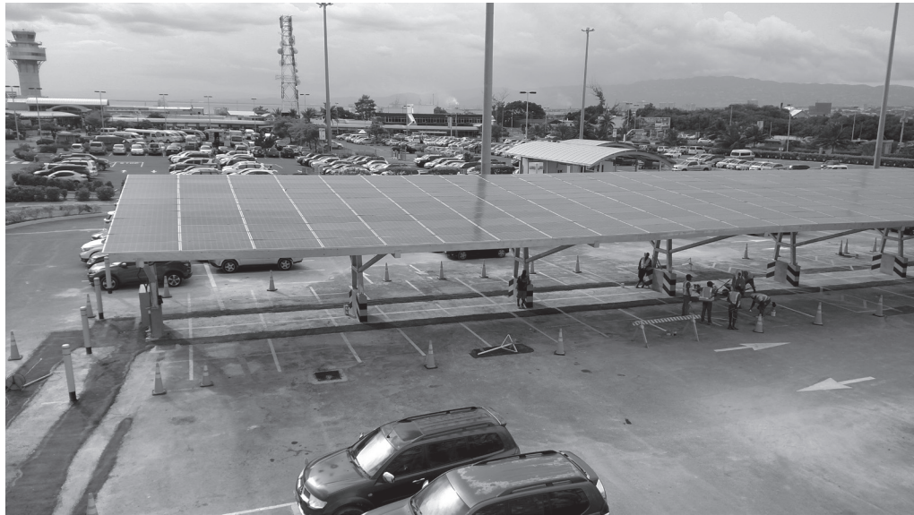
Figure 5 Solar PV project at Norman Manley International Airport, Kingston, Jamaica
