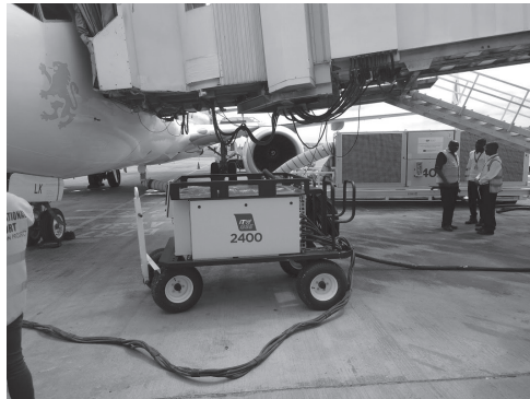
Figure 6 Gate electrification equipment at Moi International Airport, Mombasa, Kenya Source: Stephen Barrett.
